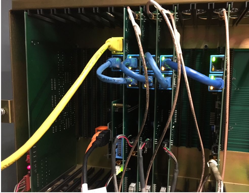
Proper connection of CAT5 cables
